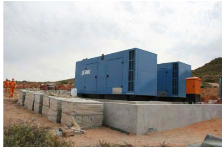
Electrical generators installed on base October 2011
